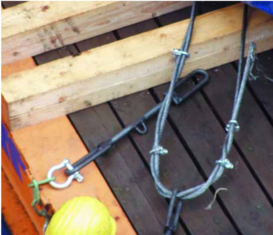
Correct lashing arrangement, not yet tightened. The steel wire is twisted to increase the friction.
